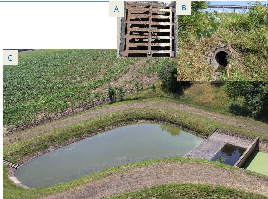
Fig. 9: Water drain on road (A), drainage system (B), and retention pond (C).
